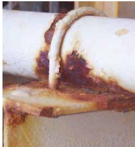
Above, the result of crevice corrosion on a pipe. Trapped moisture has caused substantial wall loss that could result in catastrophic failure.
